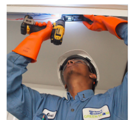
Direct installation of Energy Conservation Measures (largest direct install program in the country), ConEd Small Business Direct Install, New York, NY
